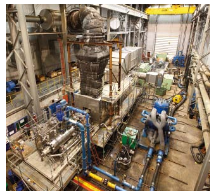
The same pump being fully string tested with gas turbine driver
